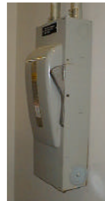
Main Power Box (S6)
